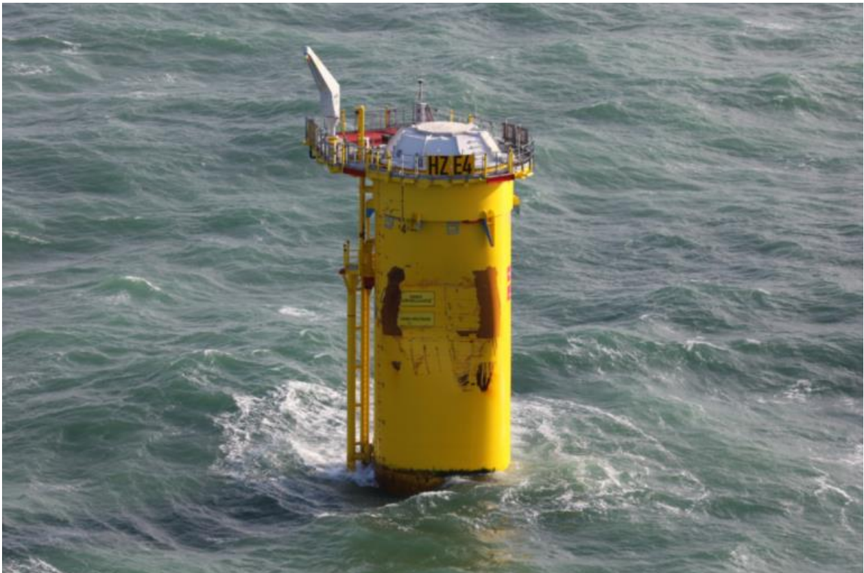
Figure 1.2 The damaged E04 turbine foundation as present in the Hollandse Kust Zuid Offshore Wind Farm, November 2023 (photo by Vattenfall).
