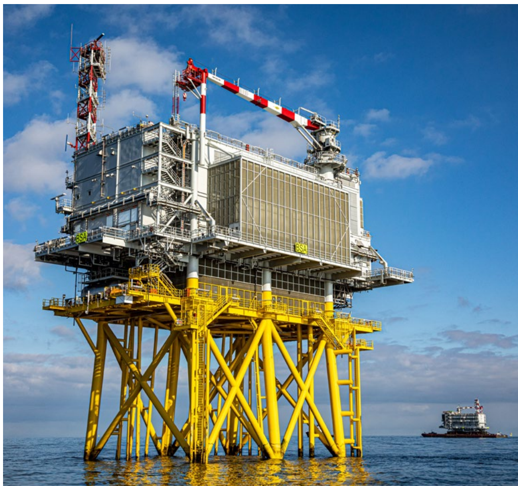
Offshore transformatorstation Borssele Beta.
