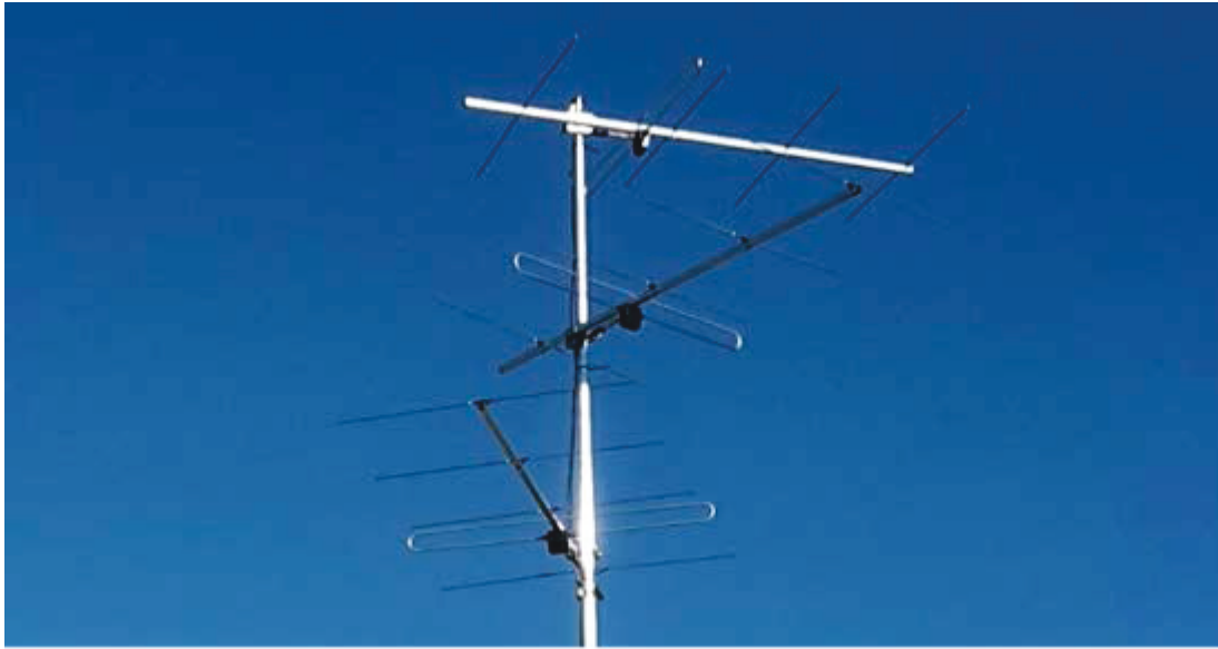
Figure 2.7: Yagi 5-element antennas rotated at an angle of 60 degrees relative to each other.
